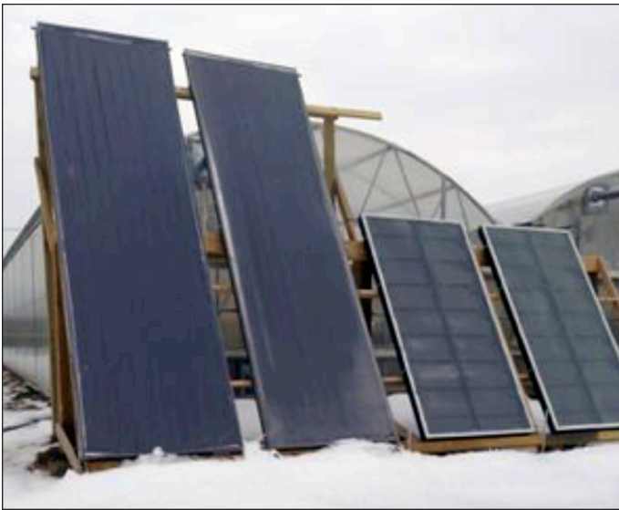
Figure 2. Thermal solar panels.
